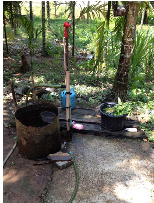
Picture 23: The water pipes (supported by Takapaw) provide some households with fresh water from the Hein Ze water reservoir (by Katharina Nydegger)
