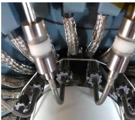
Figure 67. The cooling line electrical break in the ID end flange service region.
