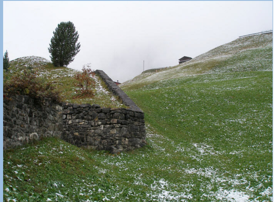
St. Antönien (Grisons), protective wall against avalanches. Photo : SLF
