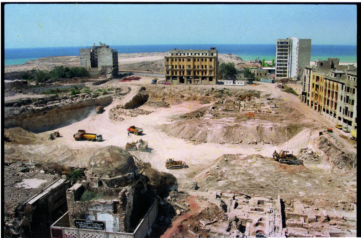
Figure 9: Beirut Souks site with L'Orient-Le Jour Building and Ibn Araaq monument. 1995. Beirut, Lebanon. © Solidere. Photograph by Mosbah Assi.
