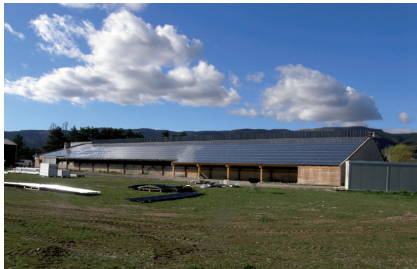
Photovoltaic plant. Baronnies Provençales Regional Nature Park. © Syndicat Mixte des Baronnies Provençales
