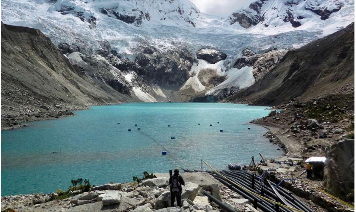
Pictured: Syphoning for lake level lowering and flood protection at Laguna Palcacocha, Cordillera Blanca, Peru. Rock and ice avalanches from the surrounding icy peaks can directly impact the lake. Photo credit: H. Frey, April 2015.
