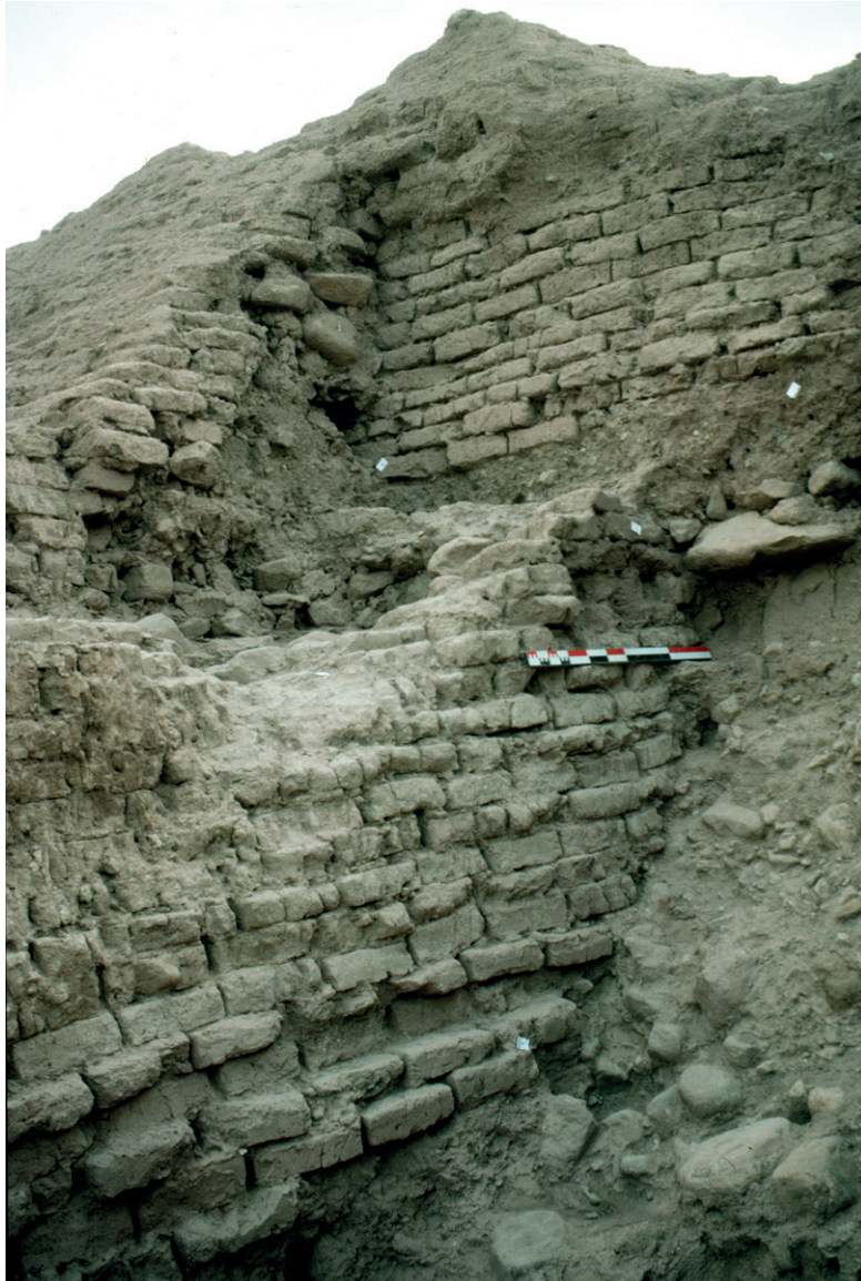
Fig. 15: Trench 4: masonry of wall and tower 2 of the Kushan period (© MAFOuz-Sogdiane 1996/C. R.).
