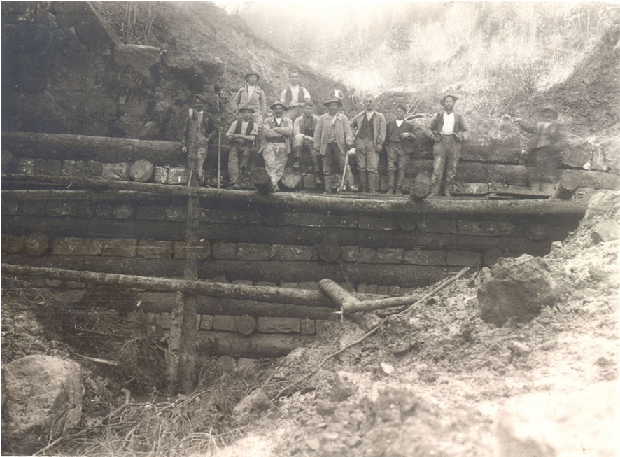
Fig. 5 Construction workers raising check dams in the gorge of the Gürbe River, ca. 1900. Copyright: Lieselotte Kappeler
