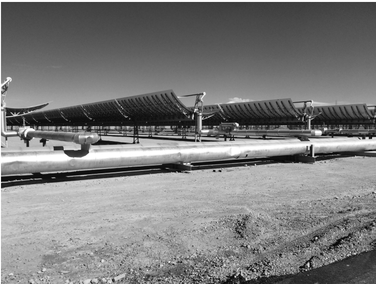
Figure 7.1 Solar panels on common land by the Solar Project Noor II in Ouarzazate, Morocco. Photo was taken by Tobias Haller in 2014.
