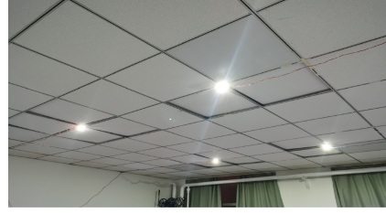
Fig. 3: LED Setup in Office
