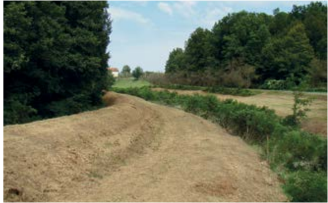
Circumferential (diversion or interception) canals to protect the agricultural area in the plain from mountain waters, Nožičko, Srbac municipality, north Republic of Srpska.
