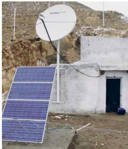
A seismic monitoring station with broadband satellite connection Location: Shartuuz, Tajikistan Photo credit: PMP International, Tajikistan
