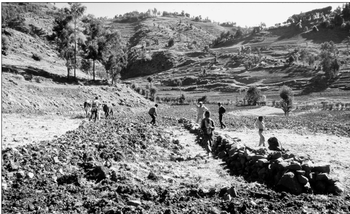
Figure 40: Moving bunds in Maybar. The stone bund has been dismantled and is reconstructed about 2 m downslope. The accumulated soil from behind the bund is distributed over the field. [Photo: E. Ludi, 1999]
