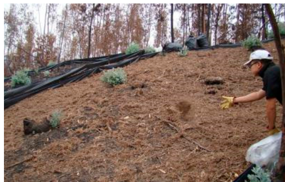
Figure 8. Spreading of natural mulch on a burned steep slope. Source: WOCAT T_POR003en, “Post-fire residue mulch”, compiled by Sergio Prats.
