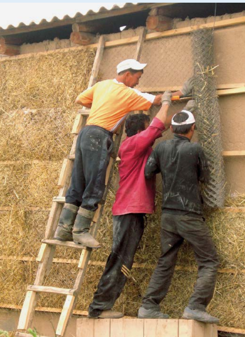
Villagers insulating a family home in Kyrgyzstan. In a better-insulated home, people use less firewood for heating; this has positive effects on their health, their household budget, and the environment. Photo: CAMP Alatau/CDE
