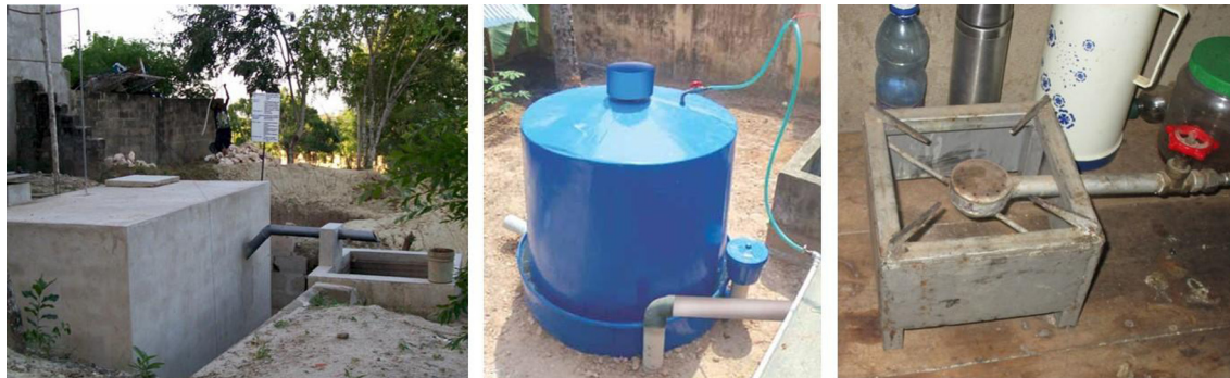
Photo 3. From left to right: VACVINA and plastic bio-digesters, biogas burner.
